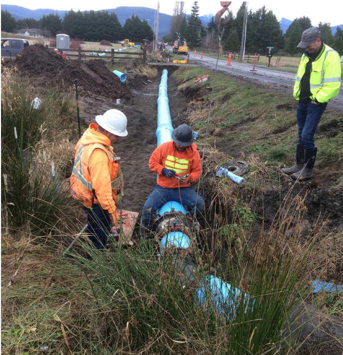
Converting open irrigation ditches to pipeline saves water and reduces the potential for sediment and pollutants to drain into waters also used by salmon. (Clallam Conservation District)
