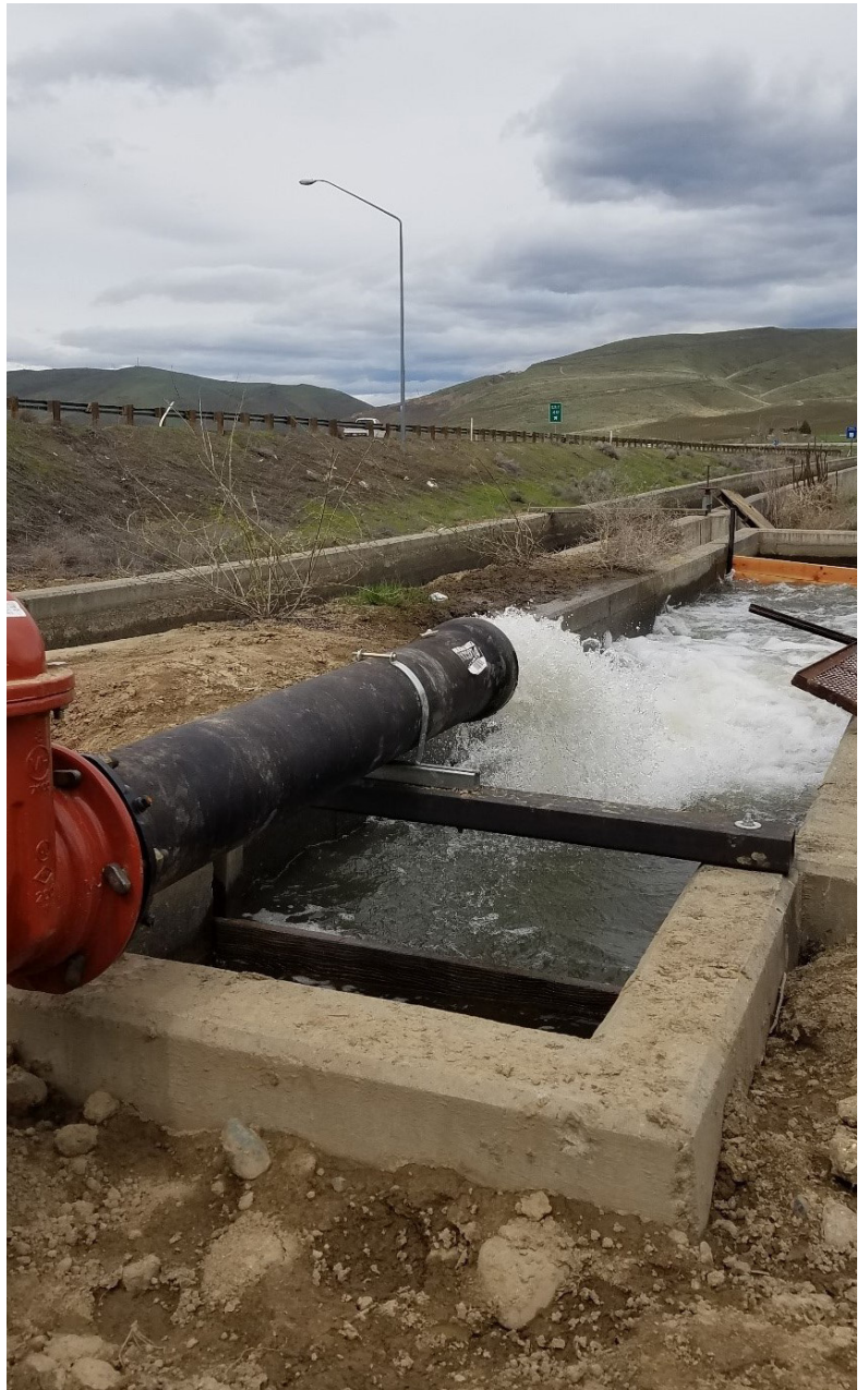
This booster pump was constructed as part of a mitigation project with the Union Gap Irrigation District to address impacts to the mainline pipe that once carried water through the Rattlesnake Ridge Landslide area.
